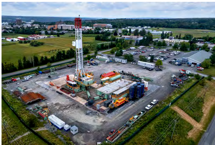
The Cornell University Borehole Observatory, located on a Cornell-owned gravel parking lot near Palm Road.
